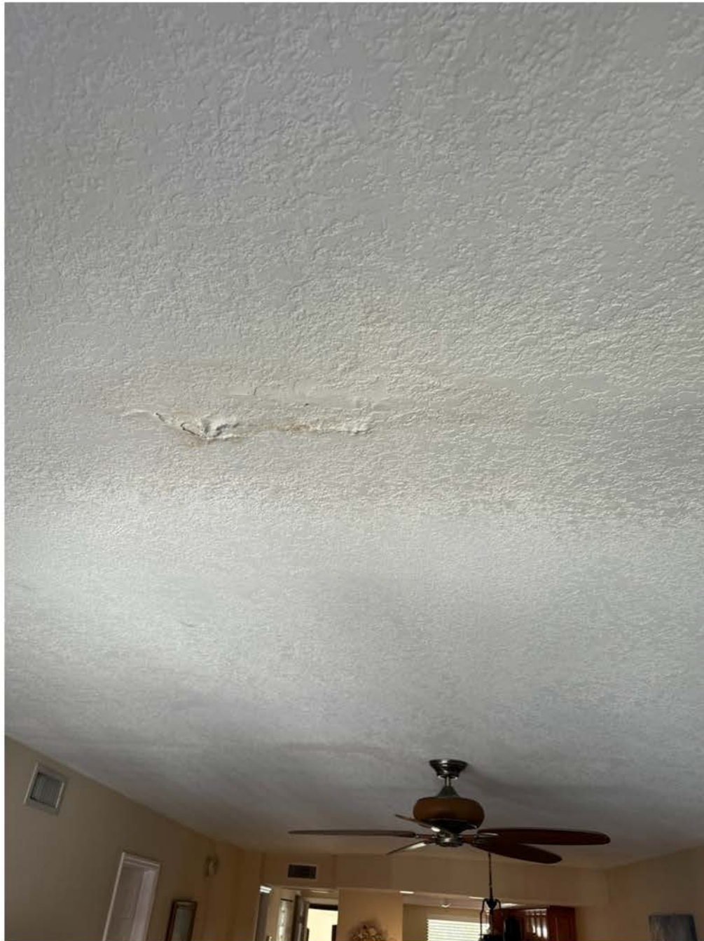
Unit 107, interior staining observed on ceiling.
