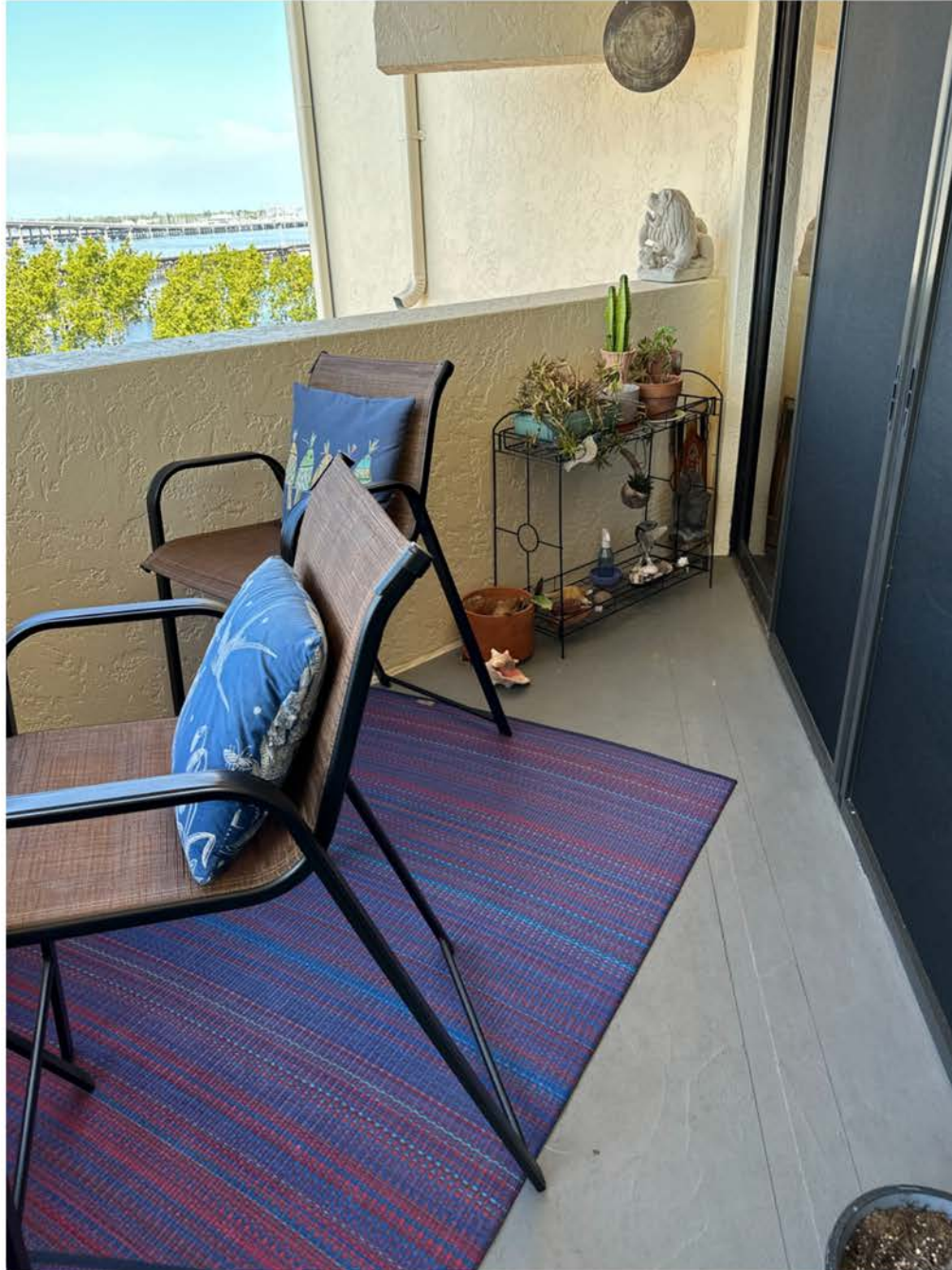
Unit 306 Balcony floor (cementitious gray finish covered in colored rugs). Appears to be in good condition, no cracking or spalling on walls or ceiling or issues anywhere adjacent that are visible.
