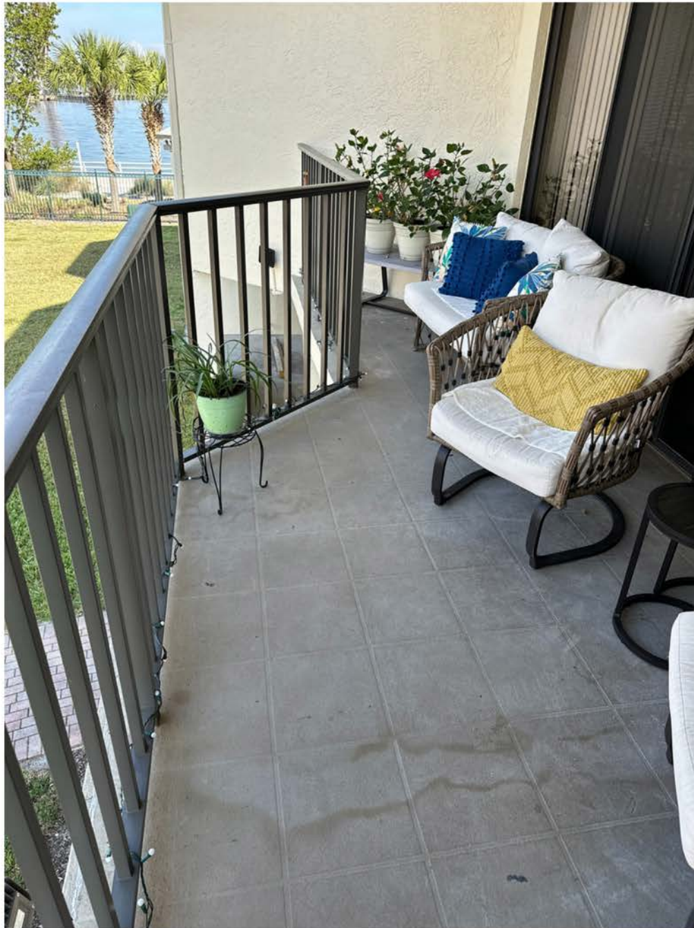
Unit 107 Balcony floor (faux cementitious tile light gray color). In good condition, with some deterioration of coating at slab edges adjacent to the guard rail post. Otherwise, no cracking or spalling in walls or ceiling. Interior drywall ceiling shows evidence of past leak, water staining. Does not appear to be an active leak.
