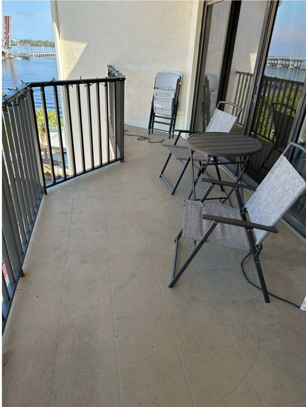
Unit 407 Balcony floor (Faux tile in brown with cementitious finish) Good condition. No cracking or issues on walls or ceiling. No action required.
