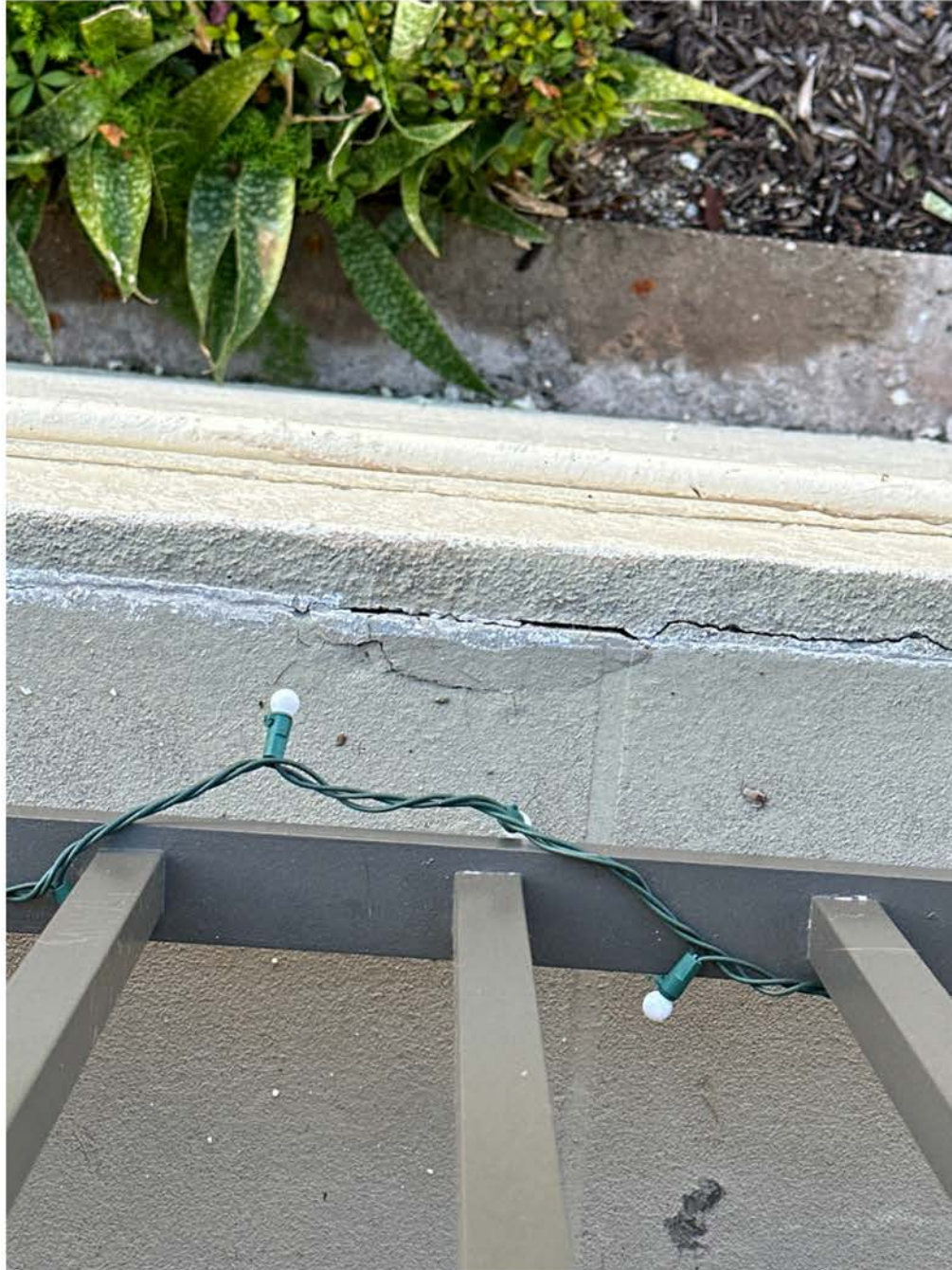
Unit 107 balcony floor at outside slab edge. Recommend investigation and repair of deck coating by licensed contractor.
