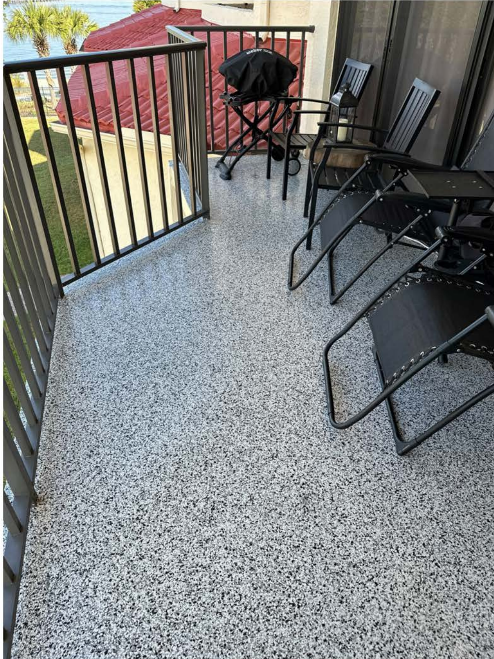
Unit 206 Balcony floor (exterior black-and-white aggregate epoxy finish) Balcony slab in good condition. No cracking or spalling in walls or ceiling or adjacent locations.
