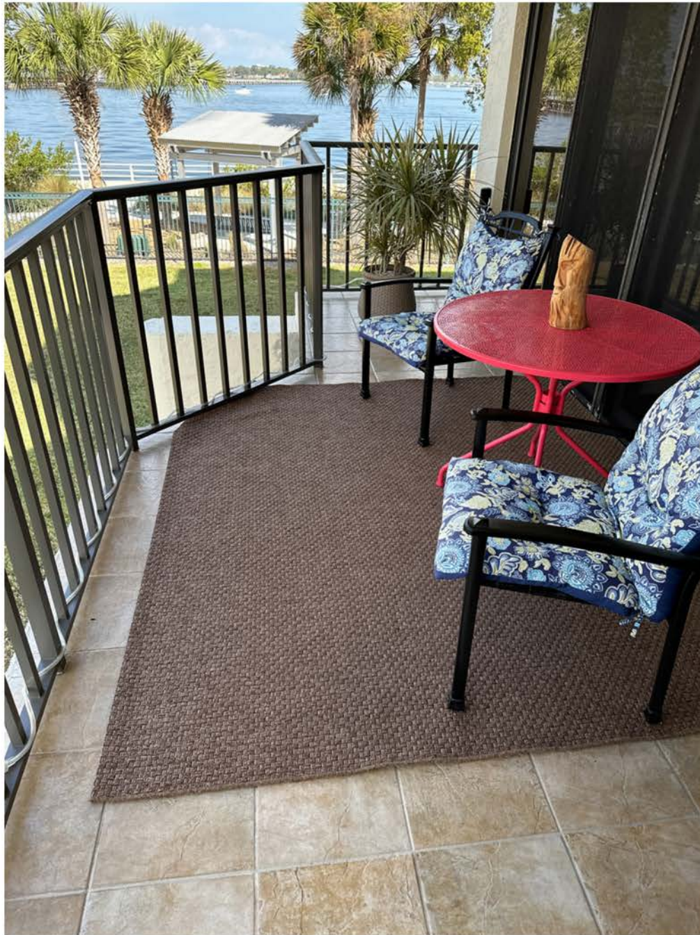
Unit 108 Balcony floor (clad in outdoor tile brown and white color mixed with area rug and chairs) Balcony slab is in good condition. No issues. No cracking or spalling on walls or ceiling. Minor cracking at balcony tile slab edge in the grout line--nonstructural issue.
